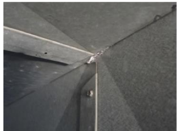
The sealant doesn't coat the duct interior but accumulates primarily in and around the leaks.
